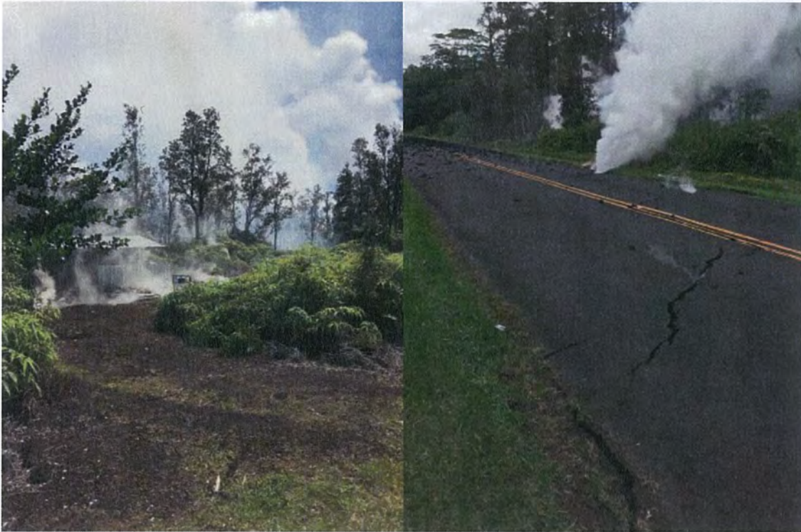
Left: Fissure 4 opened in a forest area around 10:39 a.m. HST between Kaupili and Mohala Streets. Right: Steaming cracks on Leilani Street--view is looking uprift. Crack in foreground opened during the 12:33 p.m. HST magnitude-6.9 south flank of Kilauea earthquake.
